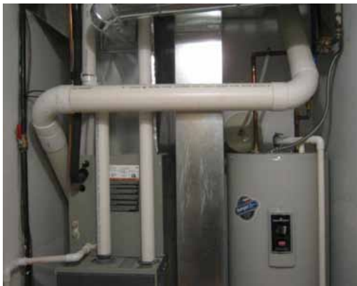
Figure 7. Example of Pipe Run Unsupported
